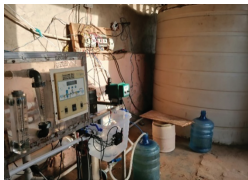
Device installed at a Water Purification Plant
